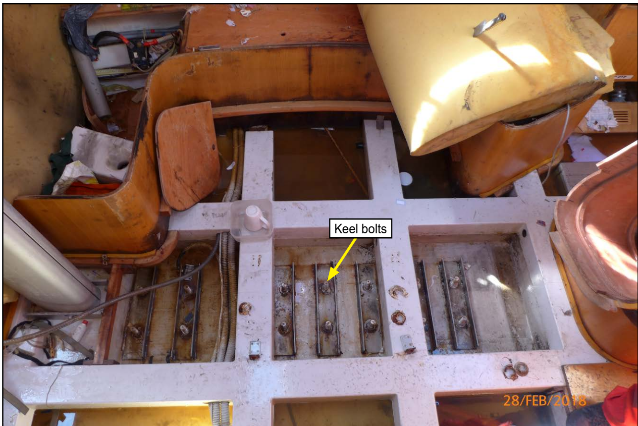
Figure 13: The keel matrix (bolts removed by surveyor prior to keel plate removal)
